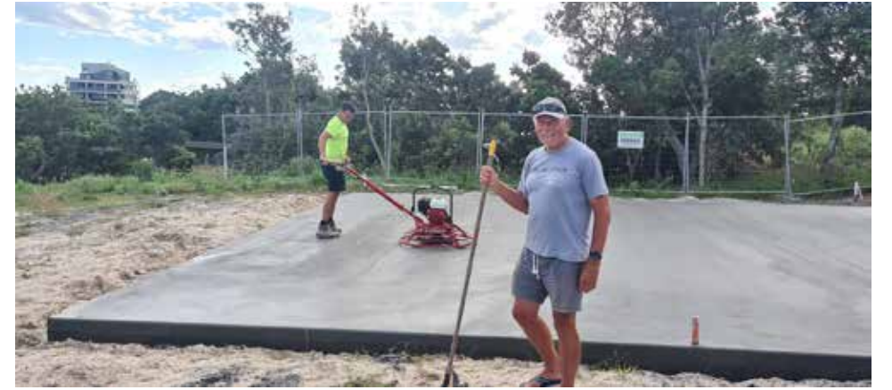
Above: Ron Hartley, proudly watching Grant Tesoriero putting the finishing touches to the concrete slab marking the commencement of Stage 1 of the new Forster Surf Clubhouse.
