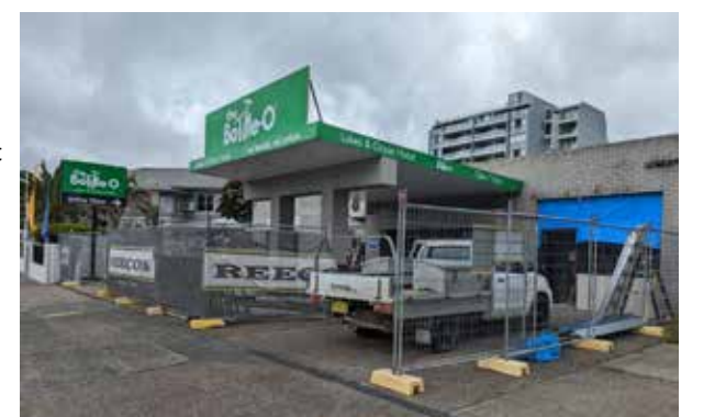
Below: Refitting a shop on Lake Street ready for The Forster Neighbourhood Centre to move in mid March.
