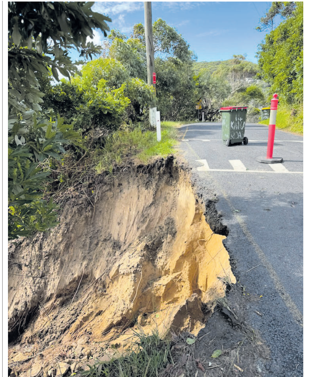
Above: A significant landslide occurred after the heavy rain at Seal Rocks on 27 April. The landslide went under the main road, down to Boat Beach. Photo by Dan Toney.
