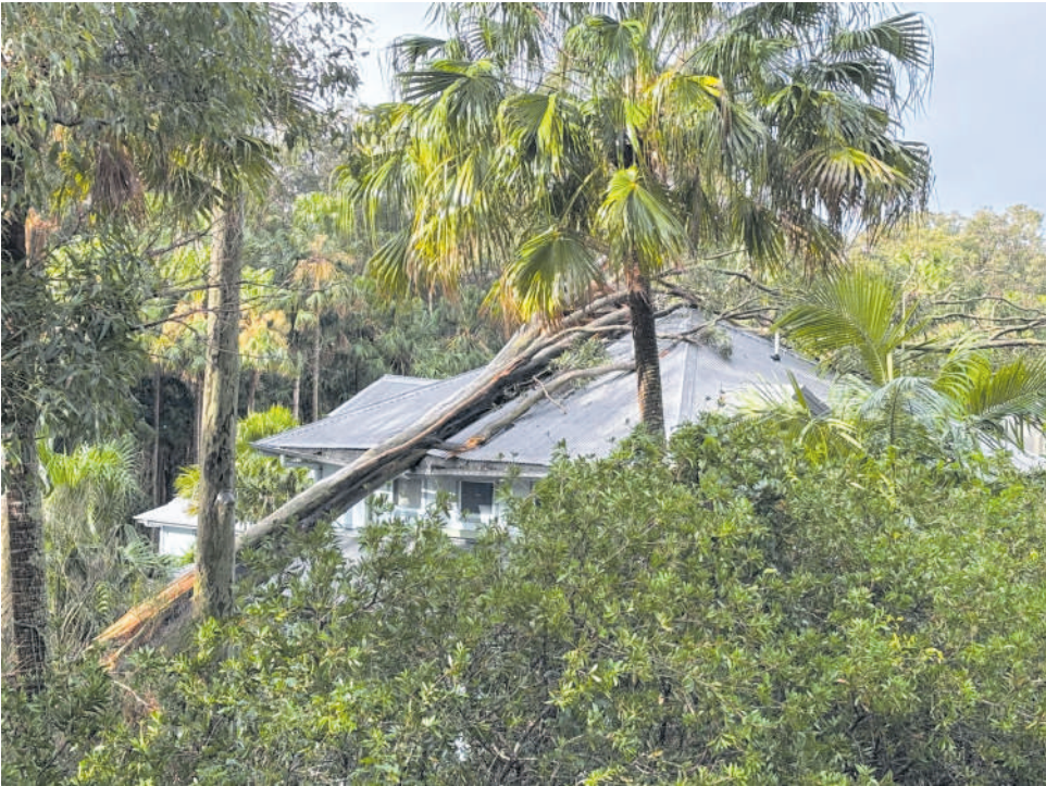
Above: A tree fallen at Pacific Palms after high winds from the coastal low during the end of June. Photo supplied.
