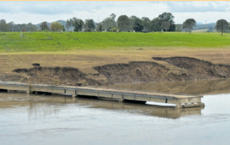
Above: Council is waiting on the engineer's assessment report on the Bight Bridge that connects Tinonee and Wingham.
