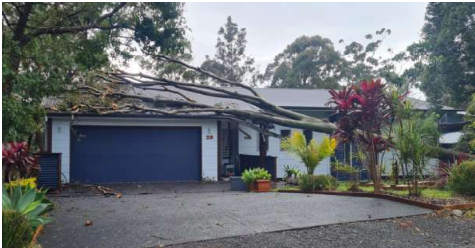
Above: Tree fallen on a house at Pacific Palms on Saturday night 2 August. Luckily no one was injured. Photo supplied.
