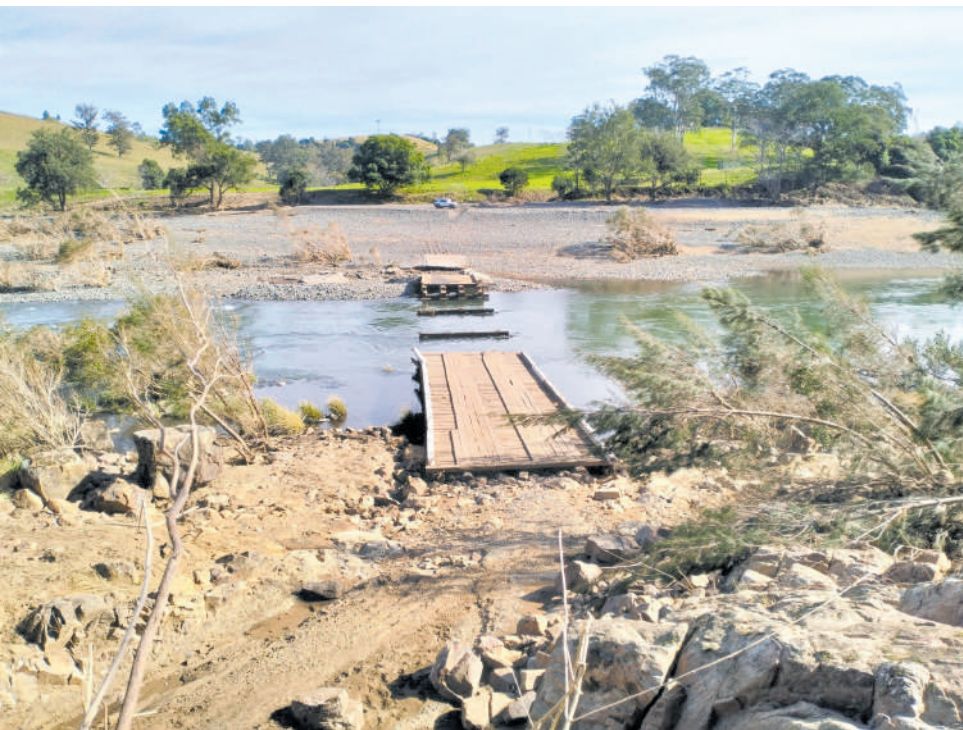
Above: A temporary solution to the Tiri Bridge issue (between Mount George and Cundle Flat) is on its way. The bridge was washed away during the May 2025 floods and there has been no functional crossing in that vicinity since.
